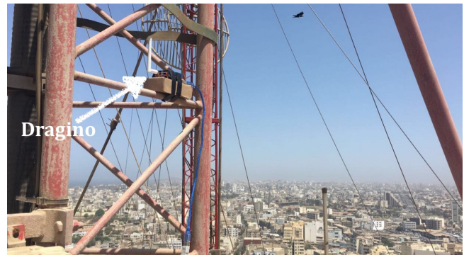
Fig. 3. A given base Station located in the highest building in Dakar.
